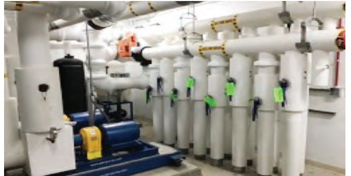
6. Right Side of Geothermal Room
