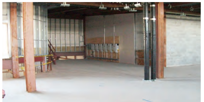
8. Solar Meters Located Off the Future Lounge and Sleeping Quarters on the 3rd Floor
