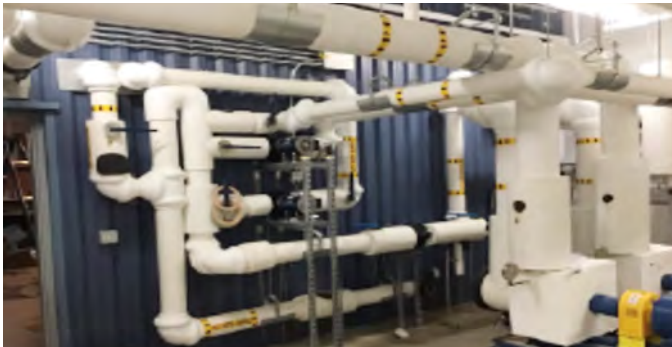
5. Left Side of Geothermal Room
